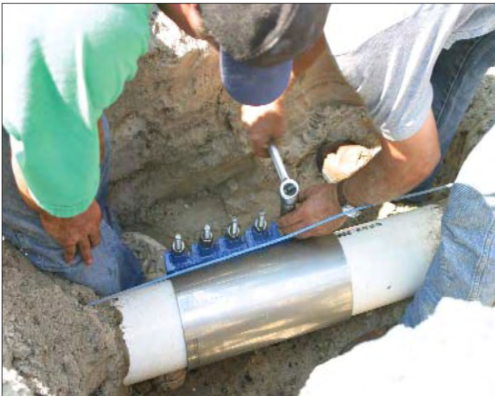
Figure 7: Vacuum sewer repair (full-circle clamp)
