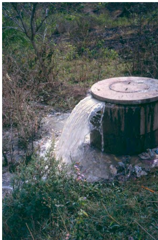
Figure 27: Overflowing manhole due to excessive inflow
