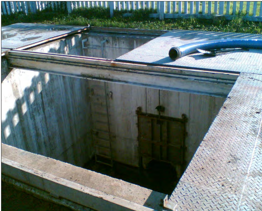
Figure 17: Sliding roof cover for silt trap (courtesy of BKS (Pty) (Ltd))
