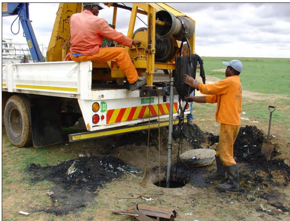
Figure 6: Cable machine for cleaning infrastructure (courtesy of Sight Lines Pipe Survey Services)
