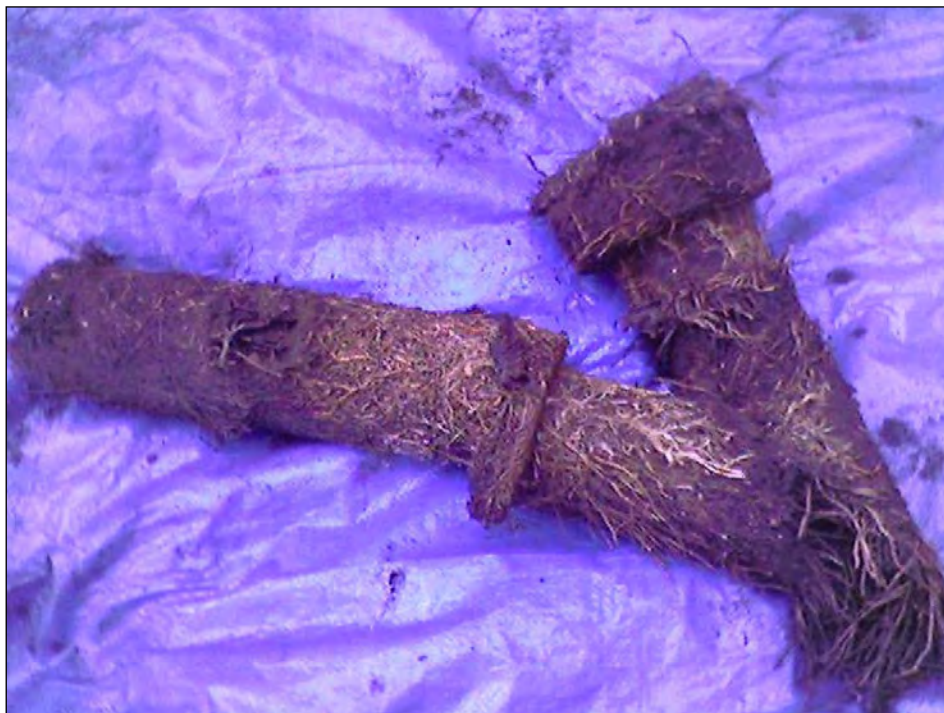
Figure 15: Excessive root obstruction
