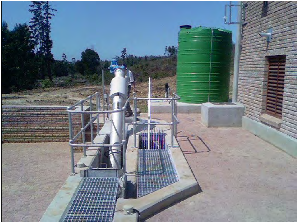
Figure 20: Combination of mechanical and manual screening devices (courtesy MVD Consulting Engineers Suid-Kaap)
