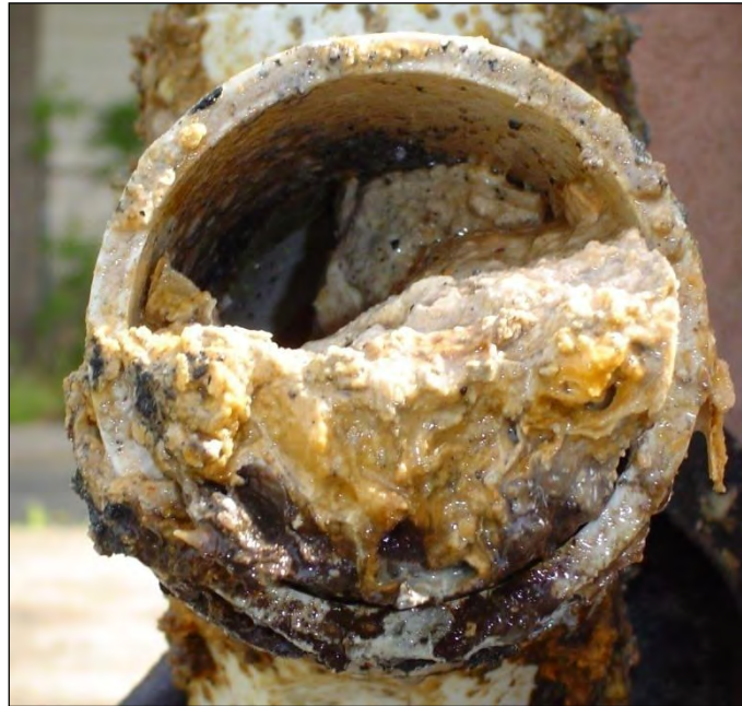
Figure 28: Grease in sewer
