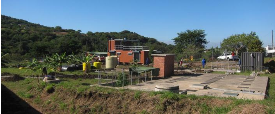
Figure 18: DEWAT trial plant
