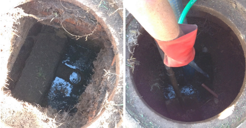
Figure 16: In tact invert level in the second chamber and watering down to loosen the sludge
