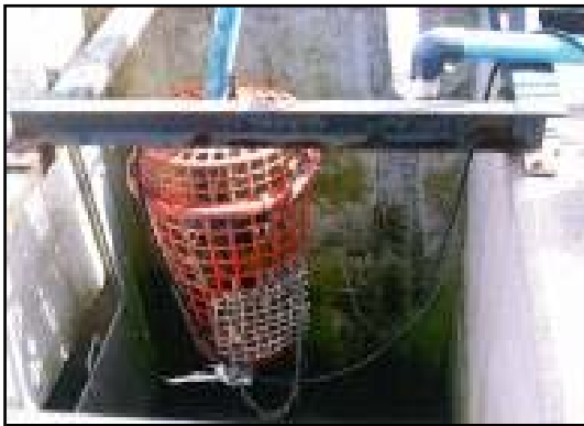
Figure 4-7: Pump housed in a meshed basket
