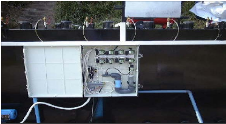
Figure 4-4: Gas measuring system for the ABR
