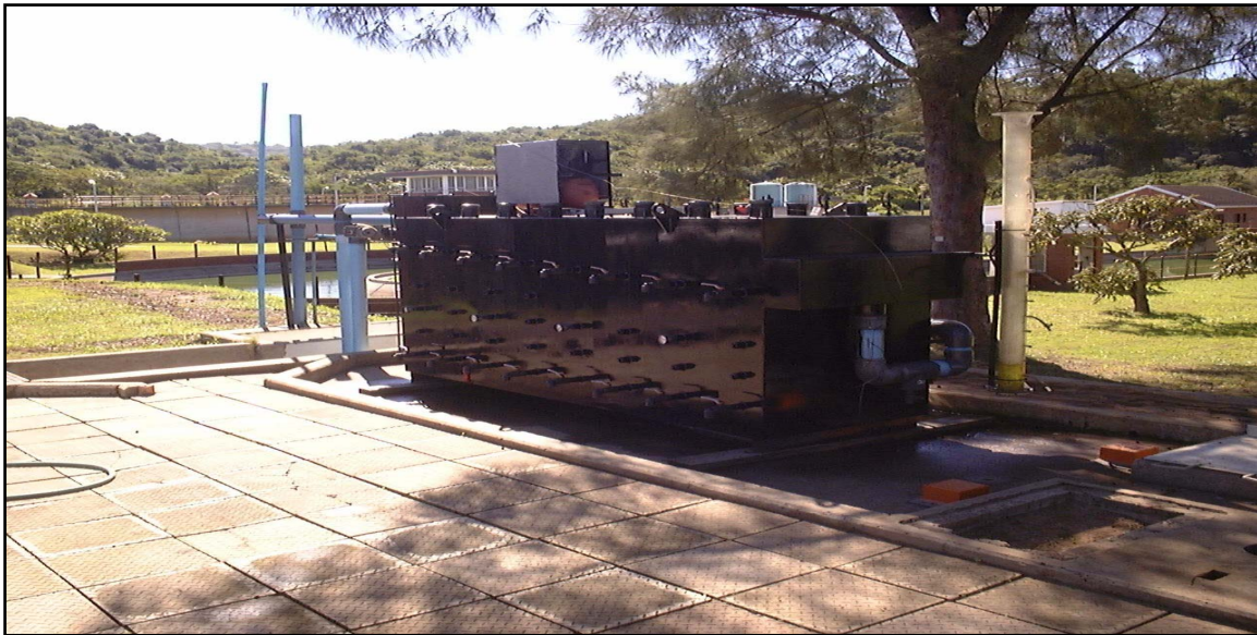
Figure 4-2: Photograph of the pilot-scale ABR at Kingsburgh WWTW
