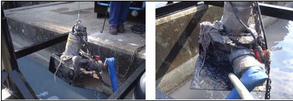
Figure 4-6: The plate proved very ineffective in preventing rags from entering the pump
