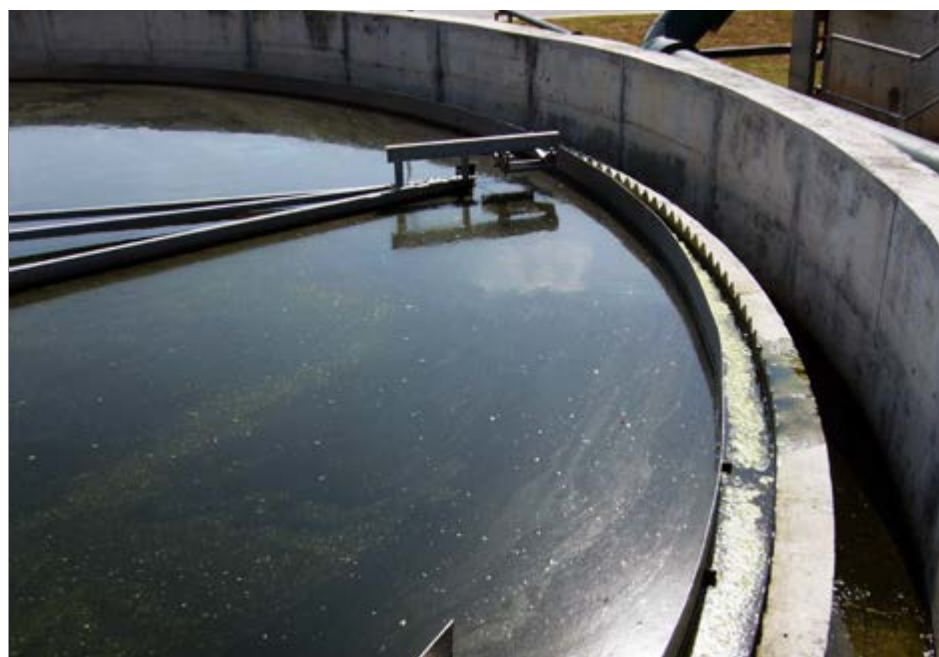
Figure 4.3 Circular sedimentation tank
