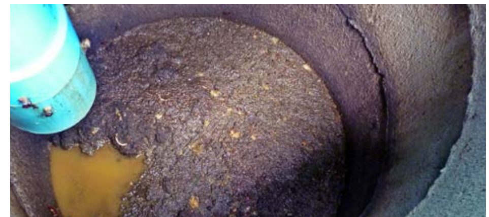
Figure 1.3 Sludge accumulation in cesspool
