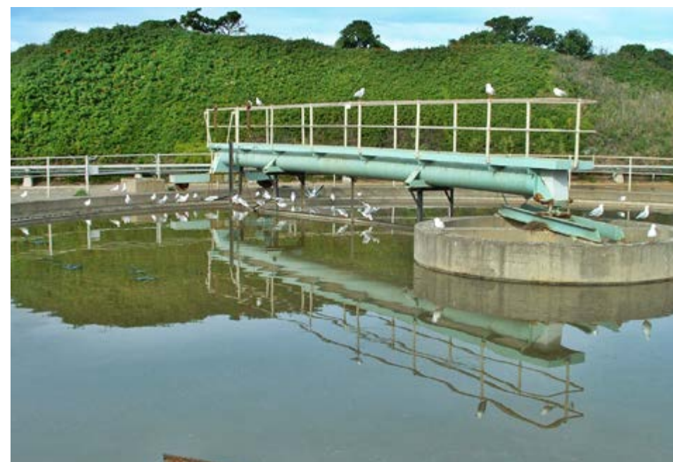
Figure 4.4 Sludge sedimentation tank
