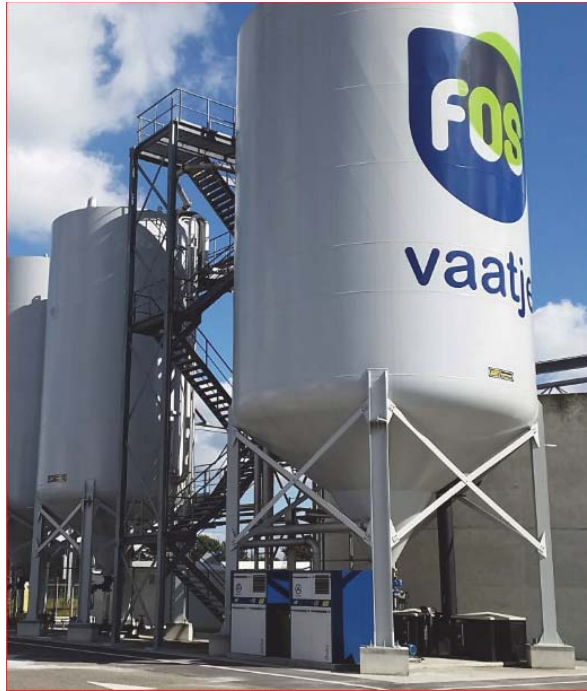
Figure 14: Struvite Precipitation plant from Sludge in Amsterdam, Netherlands
