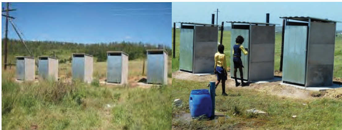
Brand-new toilets, installed by the franchisees, at two other schools.
