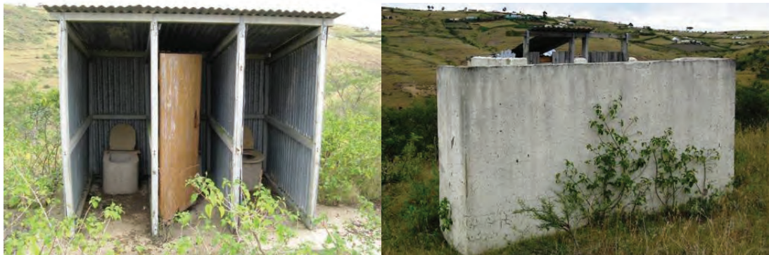
(Left). Learners' cubicles unusable -- no doors, overgrown. (Right). No roof to toilet block
