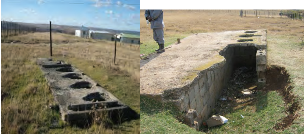
Toilets destroyed beyond repair.
