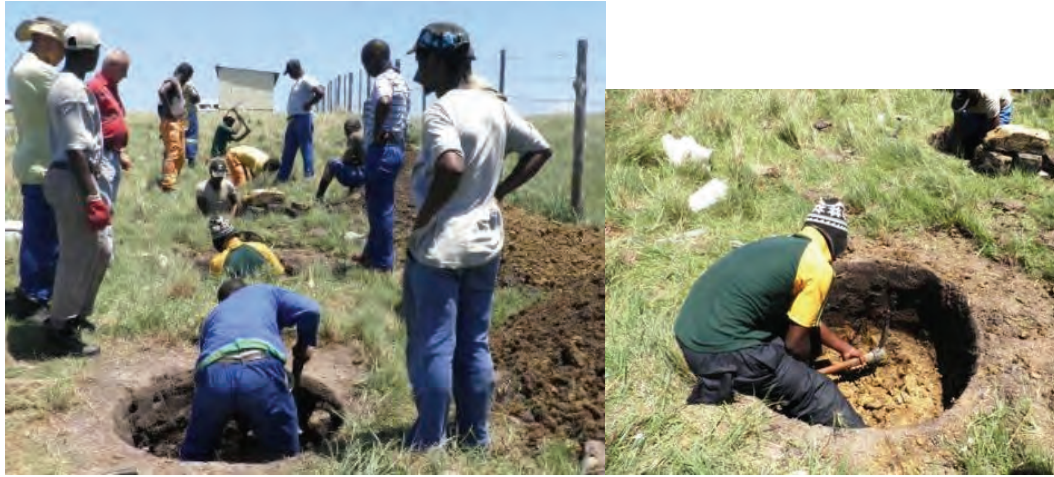
Franchisee Gary Sixaso's brother (in slouch hat, photograph left) supervising his brother's team digging holes for toilets.
