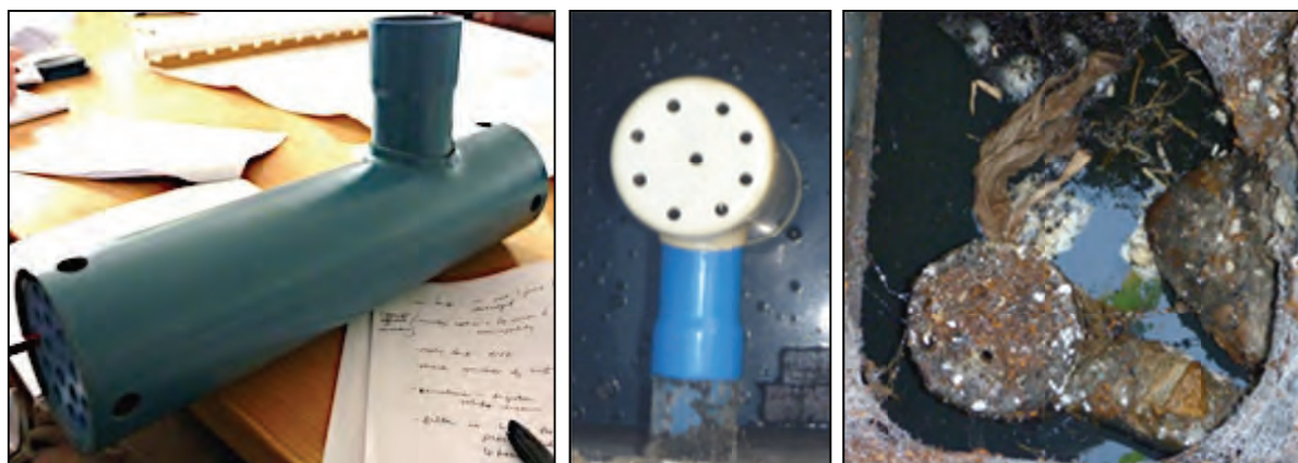
Figure 4-4: The 63 mm outlet filter (left) that is installed in Hermanus' properties. The middle photo is of a filter on a new tank that was just commissioned and the photo on the right is of a settled tank that has been in operation for several years (Photos by Ashipala (2010) and Taing (2012)).
