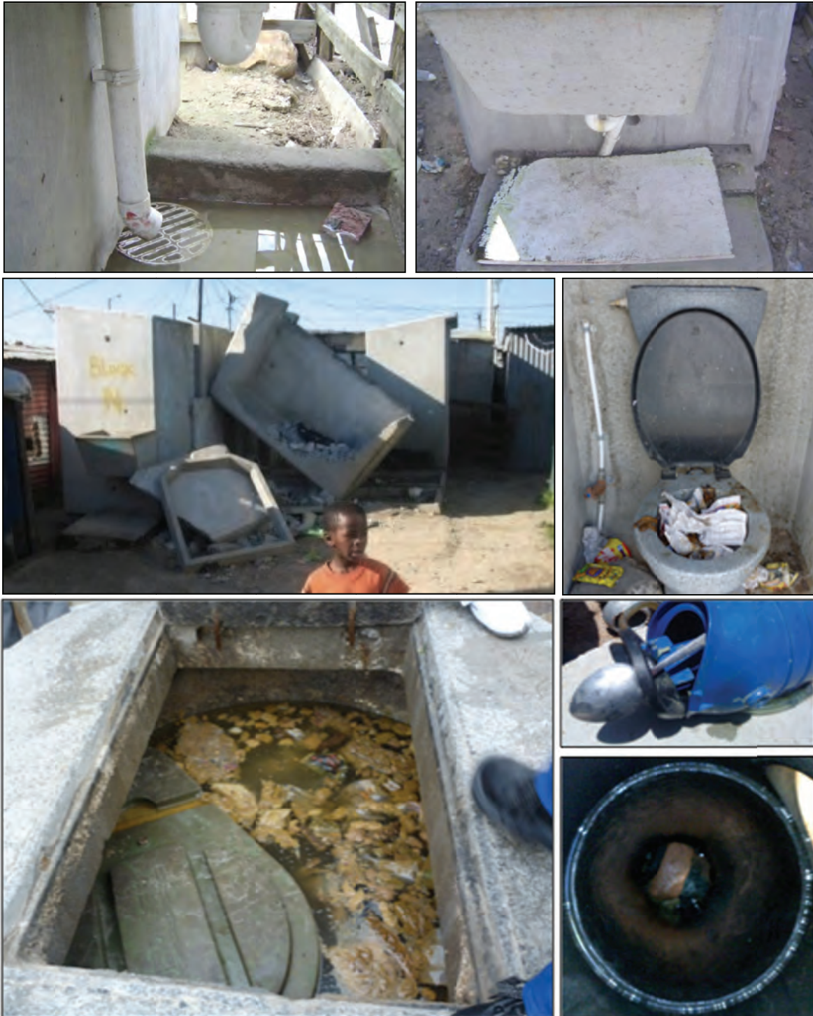
Figure 4-8: Photos of Kosovo’s vacuum system and connected toilets. Clockwise top: (a) raw sewage overflow from washbasin drain in June 2009, (b) attempts by residents to prevent spillage by covering drains with wooden boards in June 2009, (c) a used but disconnected toilet in November 2010, (d) a spoon piercing an interface valve diaphragm, (e) a brick in a sump, (f) a submerged collection chamber in a flooded concrete ring in June 2010 and (g) destroyed toilets in July 2010 (Photos by Beauclair (2009), Ashipala (2009), Cornelius (2010), Taing (2010, 2011) and Pan (2011)).
