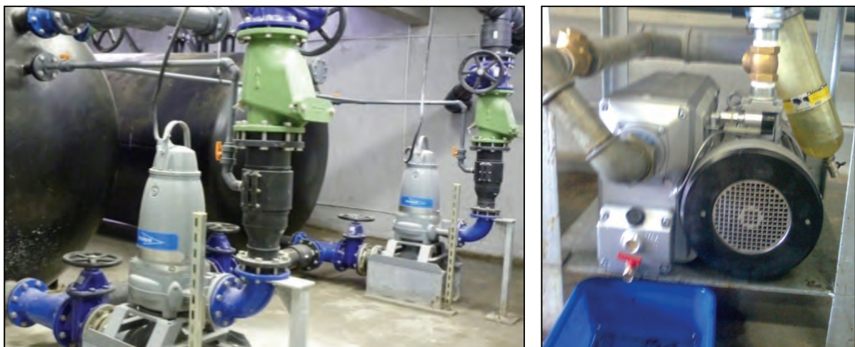
Figure B-1: Vacuum vessels and discharge pump (left) and a vacuum pump (right) (Photos by Ashipala, 2011).
