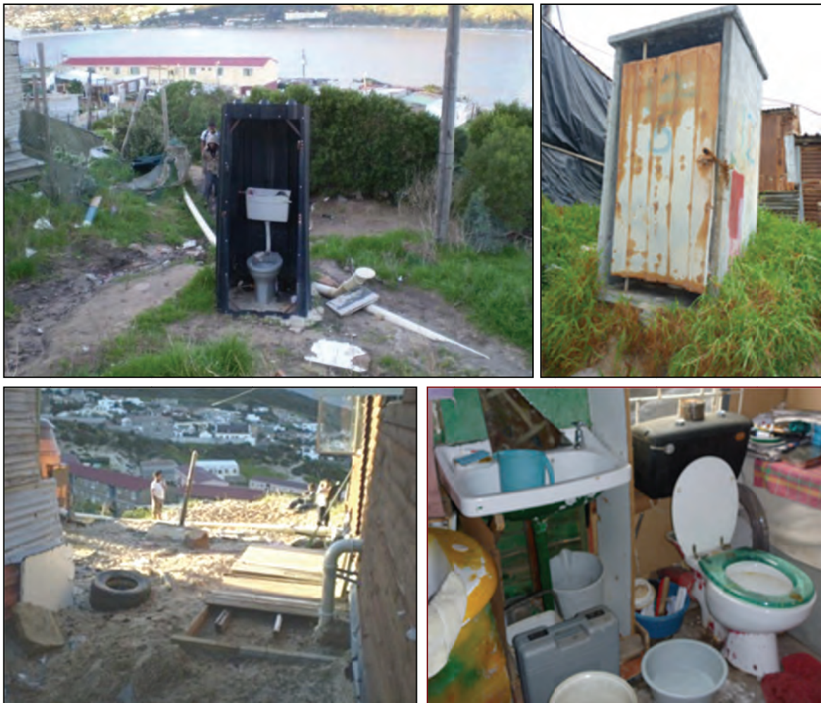
Figure 4-2: Photos of municipal and private sanitation facilities in Hangberg informal settlement. From top left clockwise: (a) a shared toilet without a door, (b) a toilet with an unstable structure due to an eroded base, (c) a bathroom in a resident's bungalow and (d) an unauthorised private connection to the exposed sewers (Photos by Ashipala (2010) & Taing (2011)).
