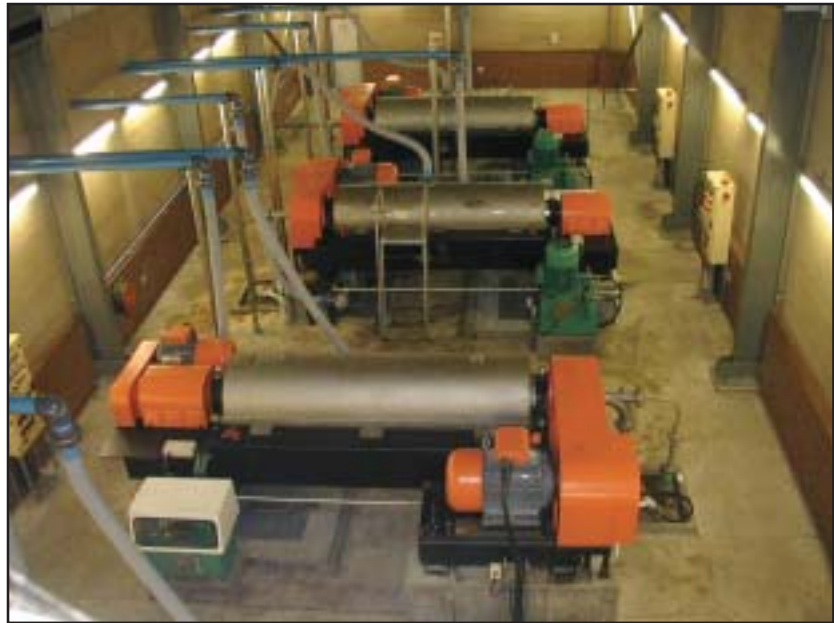
Centrifuges for sludge thickening and dewatering
