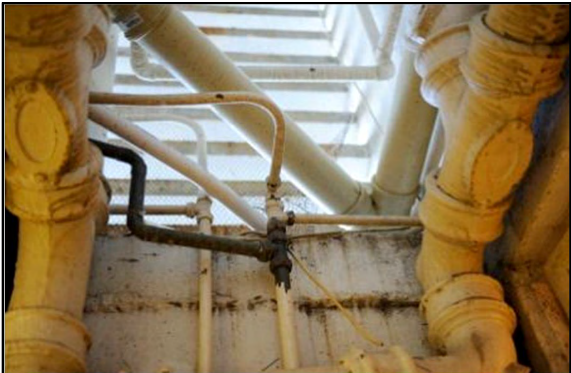
Figure 12 Retrofitting pipe work sections to accommodate collection of brown water and yellow water. Note old cast iron drains and new PVC pipe.
