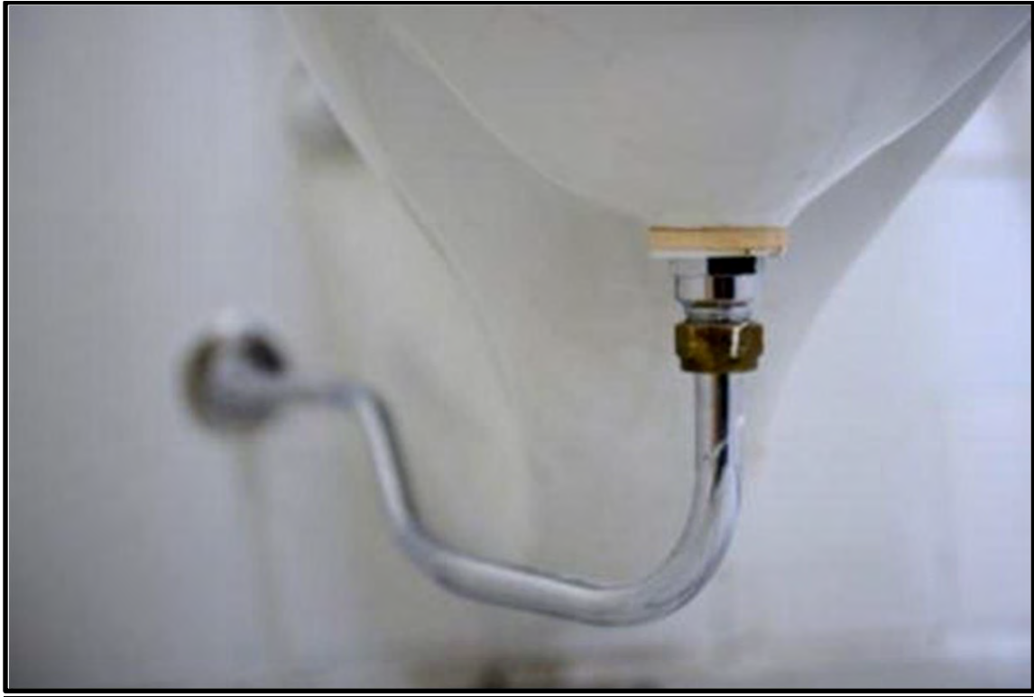
Figure 11 Stainless steel urine drain from men's no mix toilet installed at CSIR. Notice the slight bend in the pipe which acts as an odour trap.
