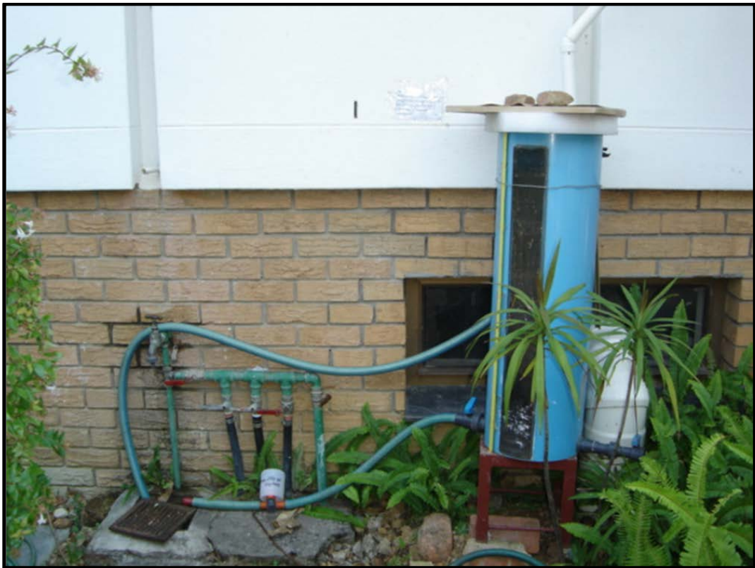
Figure 15 Grey water collection tank and pipe layout showing the inlet pipe, discharge line, overflow, and sampling point
