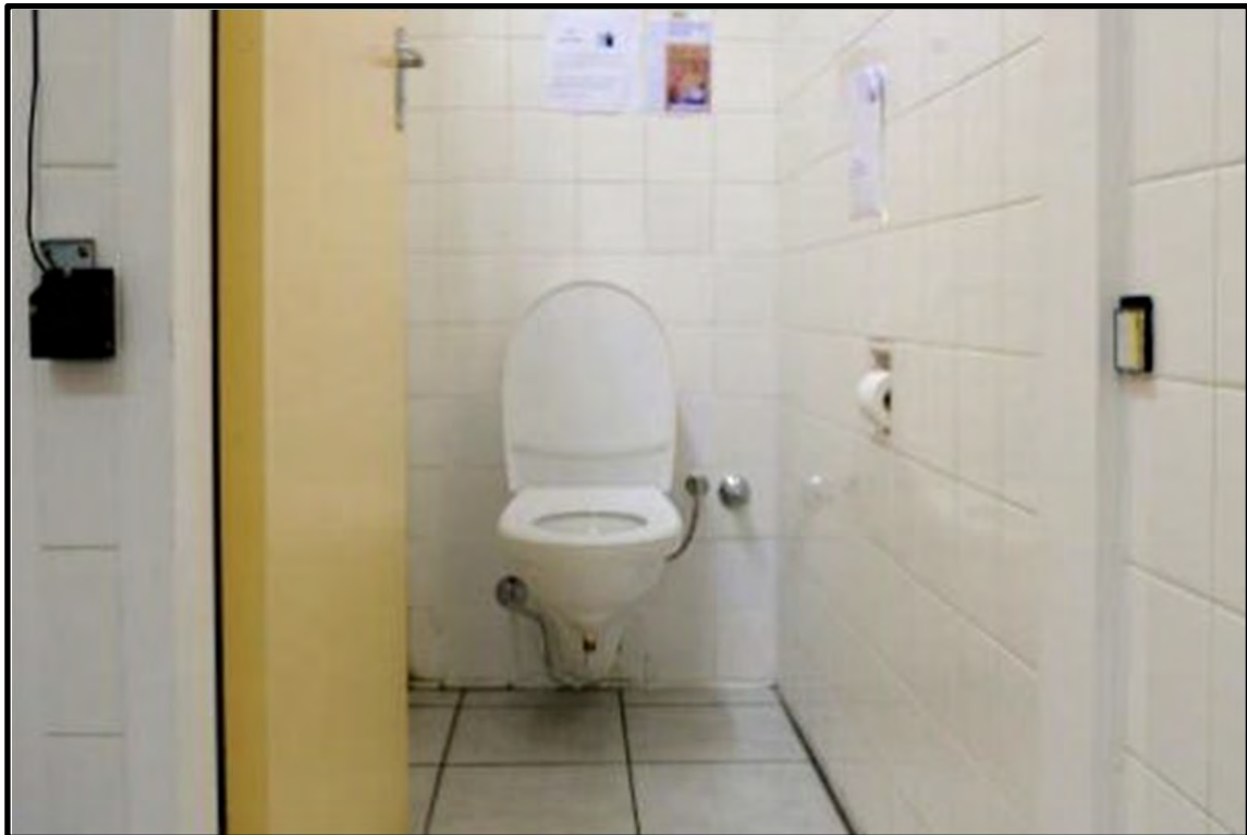
Figure 10 No-Mix toilets installed in the men's and ladies bathrooms on the 1 st floor, with an electronic counter installed to determine the number of toilet users for per person load calculations.
