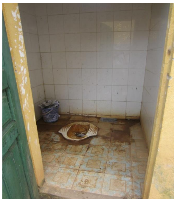
Photo 6. Composite flush latrines without water in Xa Dung communal People's Committee Headquarters.
