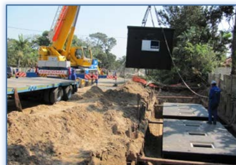
DEWATS for the Community Ablution Blocks
