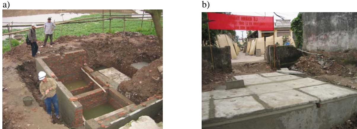
Figure 4. Baffled Septic Tank P-20 serving 20 households in Huu Hoa Commune: a) during construction; b) construction completed. (photo by Nguyen V. A., 2006)
