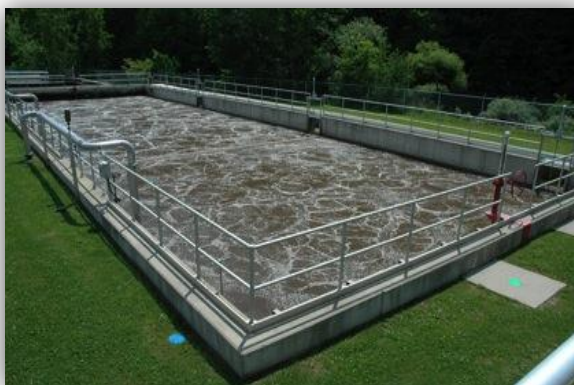
Activated Sludge/Aeration Tank
