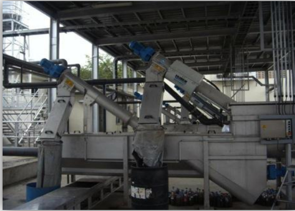
Septage Acceptance Unit
