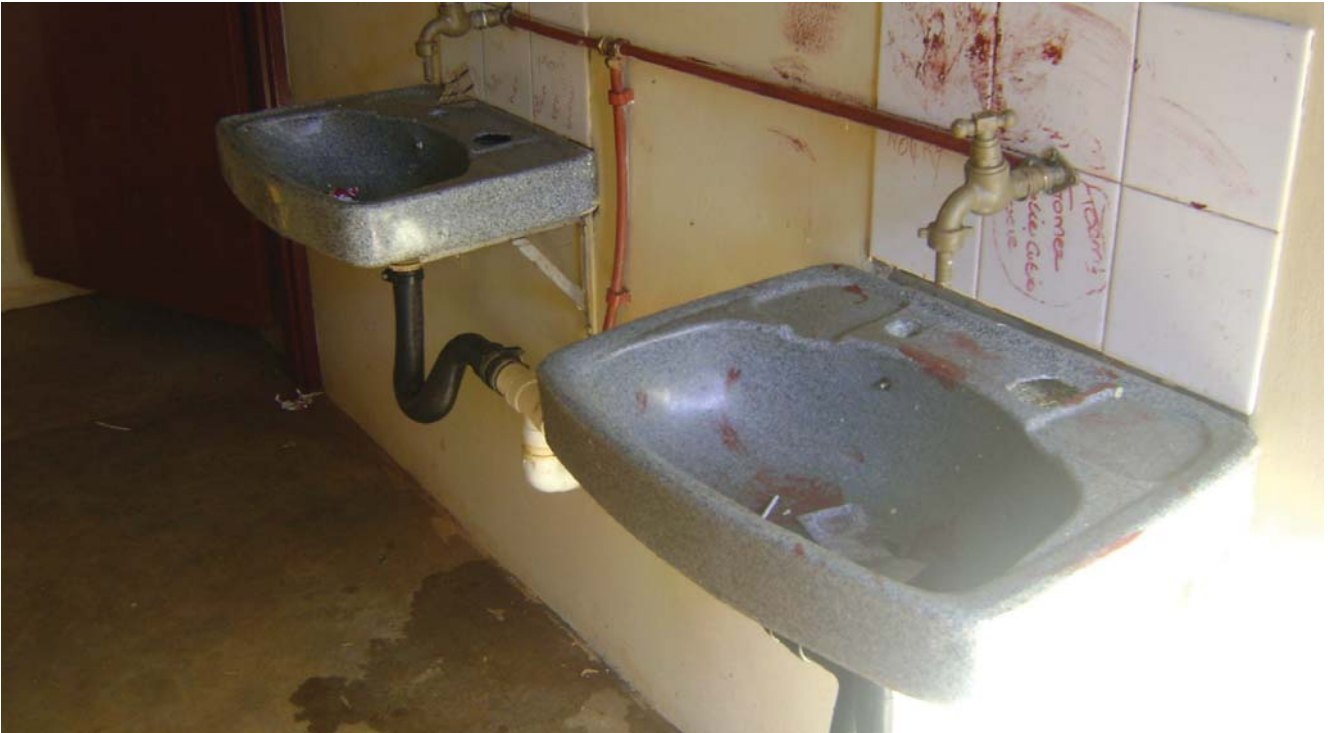
New basins installed prior to the start of the pilot programme had ready-made hole for taps, but wall-mounted taps were fitted instead. These do not extend far enough over the bowl, so water falls onto the basin ledge and then through the holes, creating large puddles on the floor. The contractor painted the walls and doors but then left behind the used paintbrushes, which learners used to daub paint on the newly renovated facilities.
