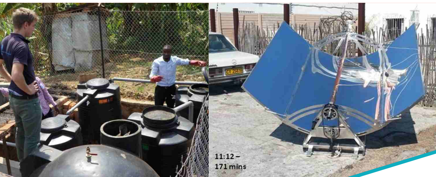
Decentralised anaerobic plant for pit emptiers to reduce transportation costs (Photo: Water for People, Uganda)
