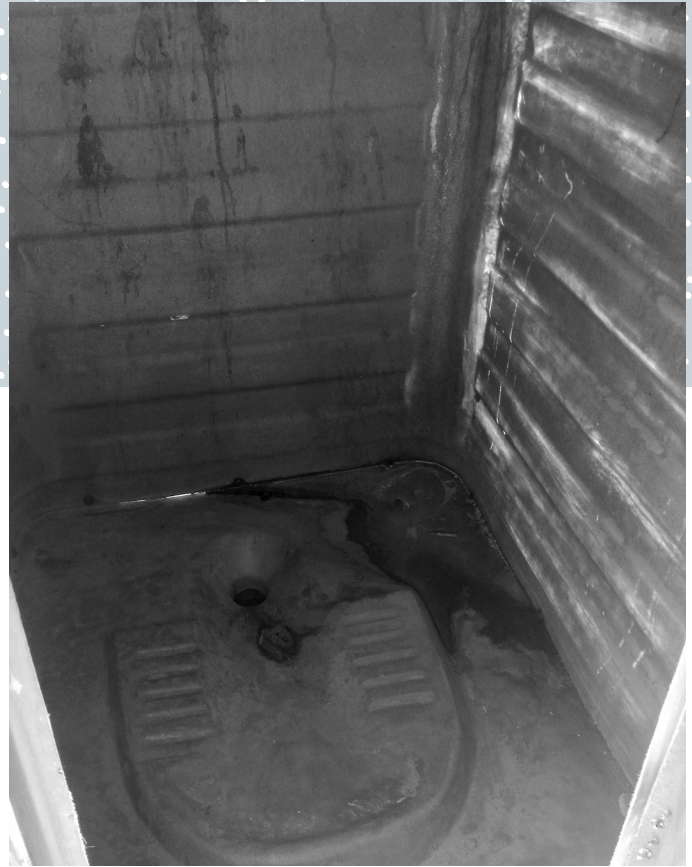
Figure 20: An Ill-maintained Individual Household Toilet
