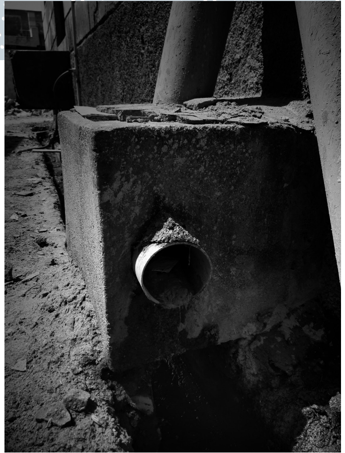
Figure 39: Insanitary Toilet, Directly Ejecting Faecal Matter into Storm Drains
