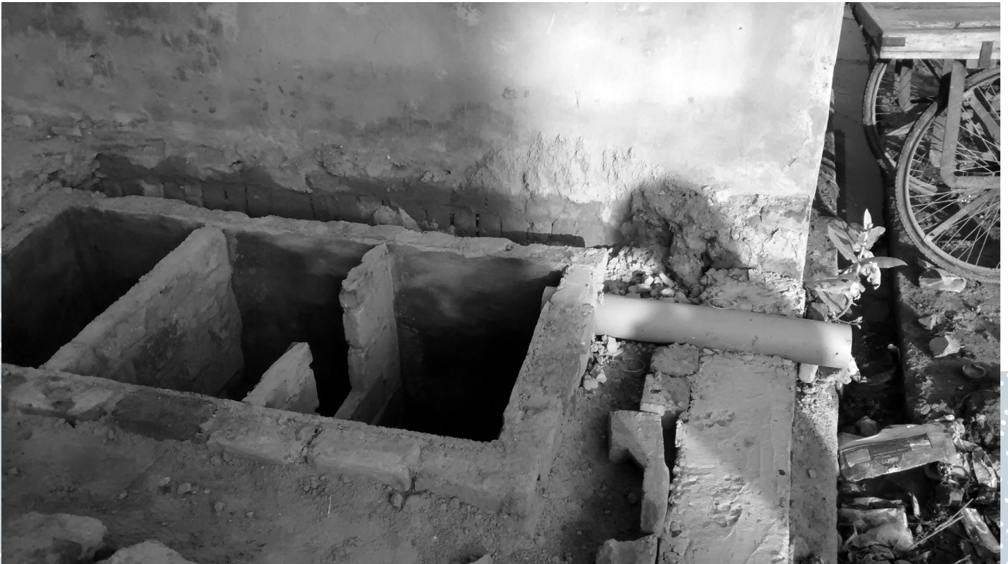
Figure 24: A Three Chamber Lined Tank with Outlet for Supernatant
