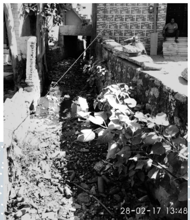
Figure 37: A Drain Blocked by Solid Waste
