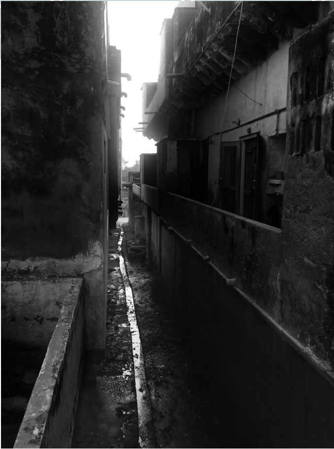
Figure 38: A Drain with Blackwater from a Series of Houses with Insanitary Toilets
