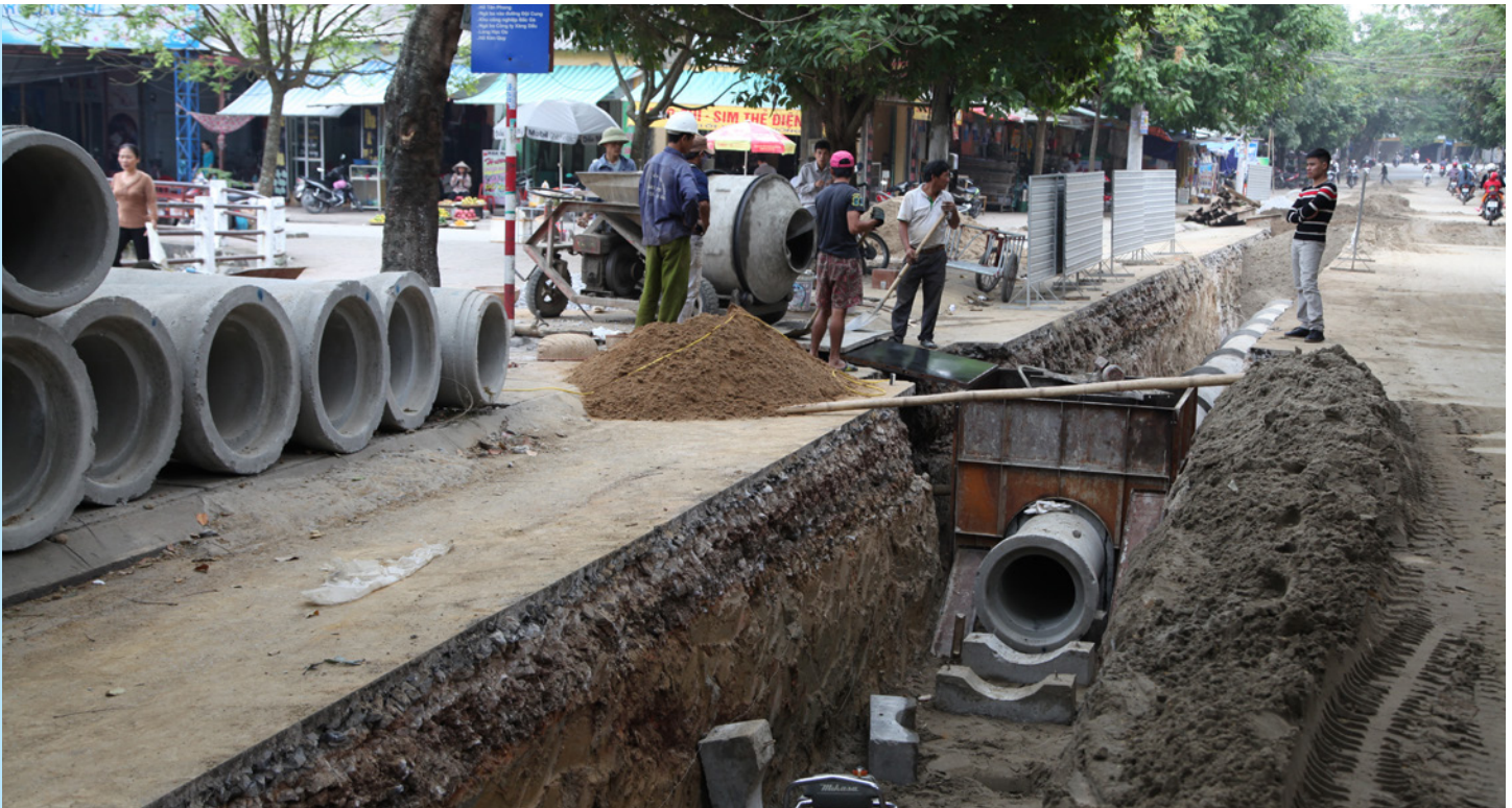
Laying pipes for a wastewater collection network brings excavation and road closures, disrupting urban life
