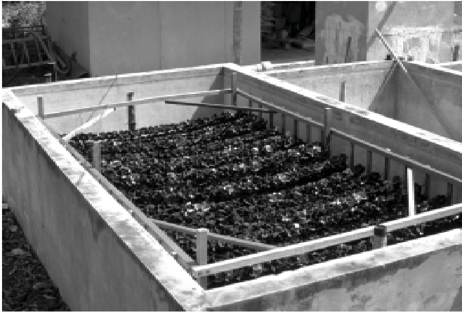
Plastic modules in the attached-growth waste stabilisation ponds at AIT, Bangkok. The ponds are used to polish the percolate from the planted septage drying beds (Photo: Thammarat Koottatep)
