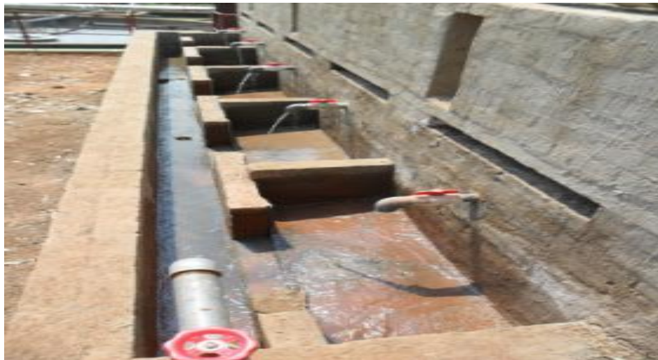
Figure 4. Basins and waste channel with a bypass outlet option in the left hand bottom corner of the multi-engineered system constructed at Kingsburgh, Durban.
