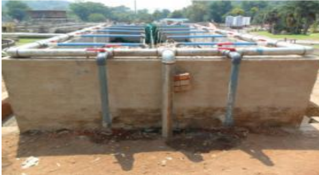
Figure 3. Front view of the multi-engineered system. The middle vertical pipe comes from the tank. The vertical pipes on the left and right are the pipes to the bottom inlet for subsurface flow. Small pipes on top of the bed along the wetland are for vertical flow, while those of surface flow are at the inside front of the system.
