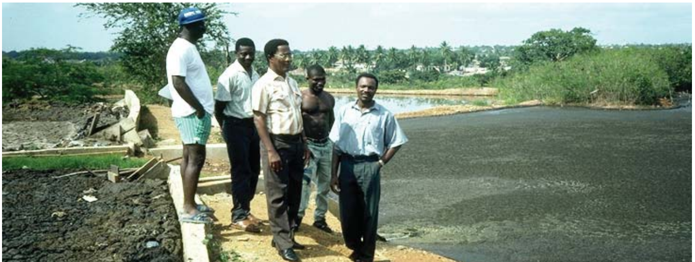
Photo 5: Ghanaian sanitation experts and treatment plant operator at an FS treatment plant in Ghana (left: FS settling-thickening tank; right: stabilization pond for settling tank supernatant)
