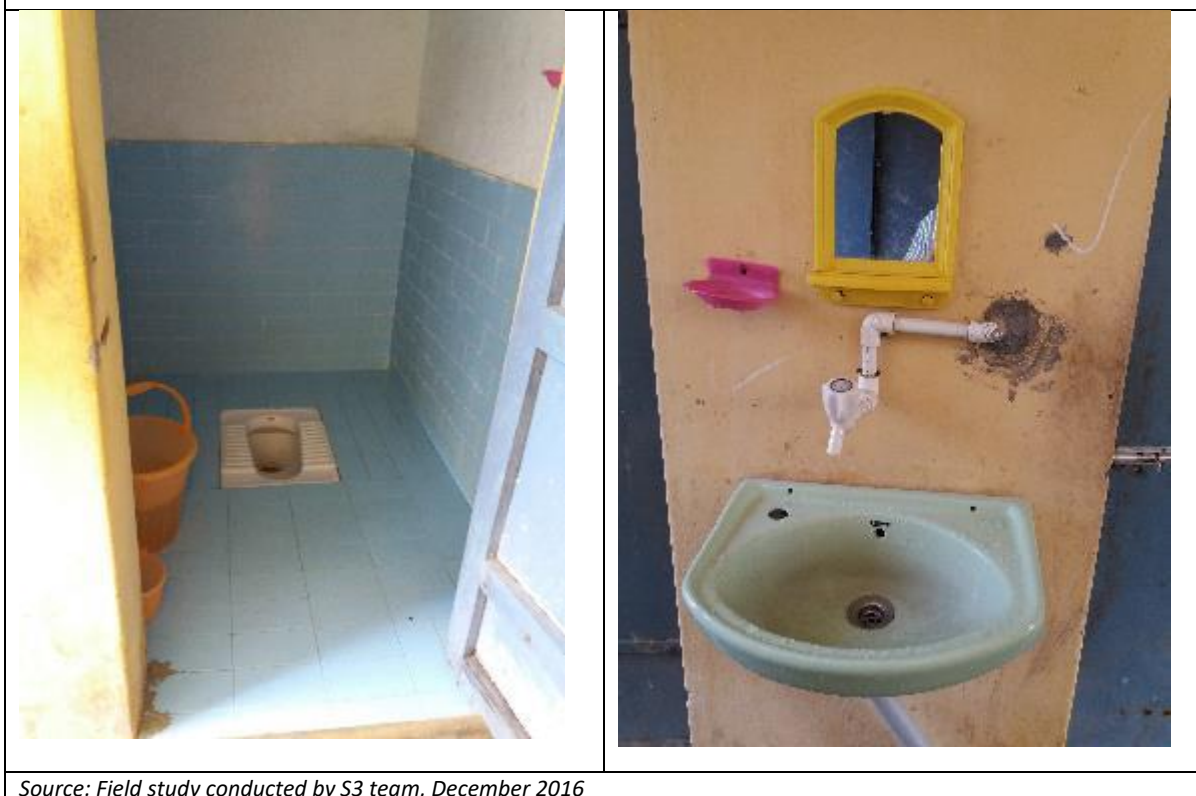
Photo 2-4 State of sanitation in Municipal high school, Kovvur
