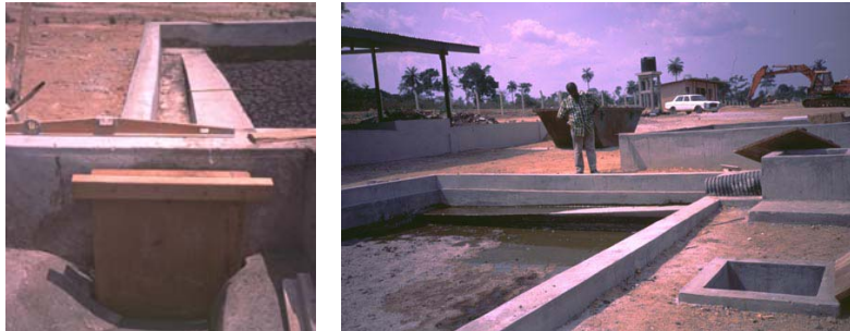
Figure 4 Inlet distribution channel (from the storage tank to the drying beds) and sludge loading
