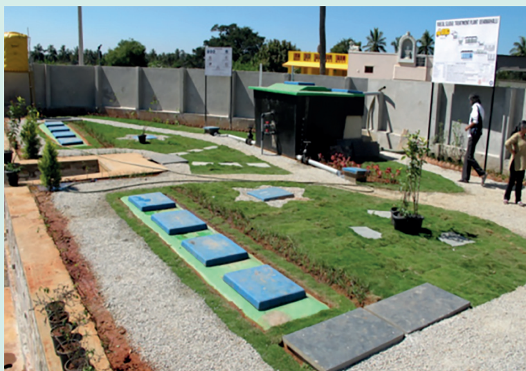
Figure 7: FSM treatment plant in Devanahalli, Bangalore
