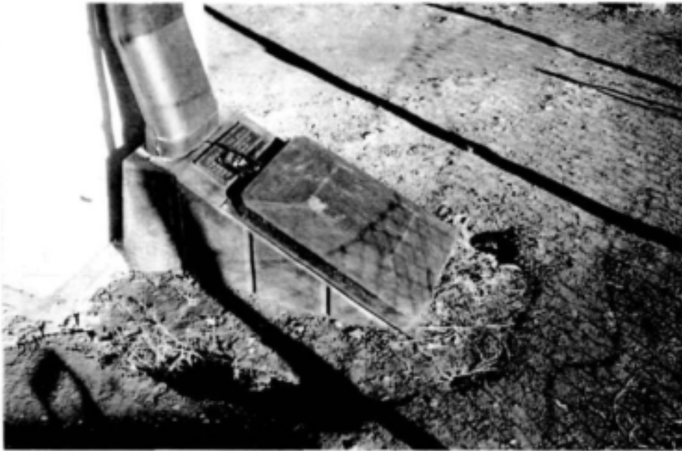
Photograph I : Subsidence of ground around Enviro Loo latrine container
