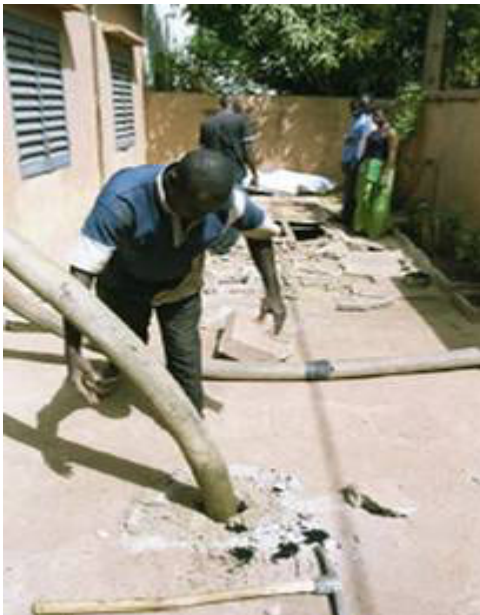
Figure IV-5: A GIE Sema Saniya septic system emptying crew works on household unit. In the foreground, the pick-axe used to break open the tank is visible across the ground. Then, a number of large hoses and extensions are connected together and strapped together using old strips of rubber. In the background, another section of the tank is open and will be pumped as well in order to assure complete cleaning.
