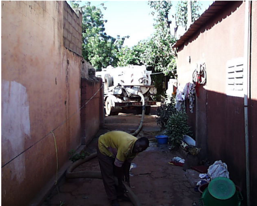
Figure III-4: Mechanical emptying of a septic tank in Commune VI of Bamako. Because of the long distances often found between the street and the pits emptied, a series of tubes must be connected together before pumping can begin.
