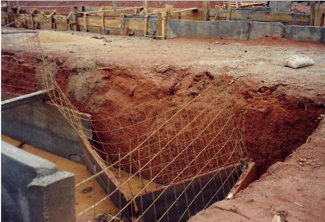
Figure VII-13: A major problem during construction was the fact that the pouring of concrete walls of the settling tanks took much longer than expected. Rainy season arrived, and unsecured walls (the gap between the hole and the walls was not filled in) buckled under the pressure from runoff. This happened in the left tank.
