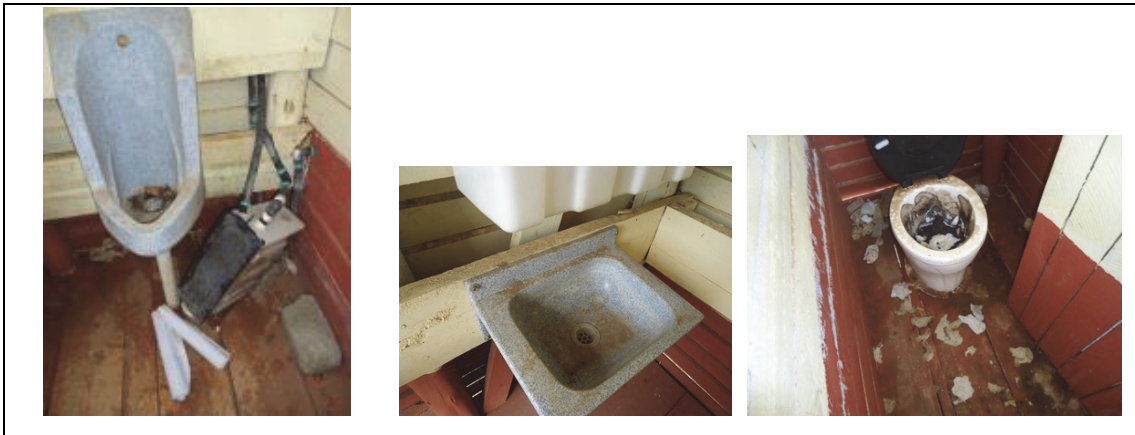
Fig 12: Examples of dysfunctional toilet, unused blocked urinal and dirty sink from the 2 Limpopo High schools
