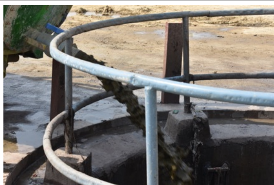
Manhole for receiving Septage at Bingawan STP
