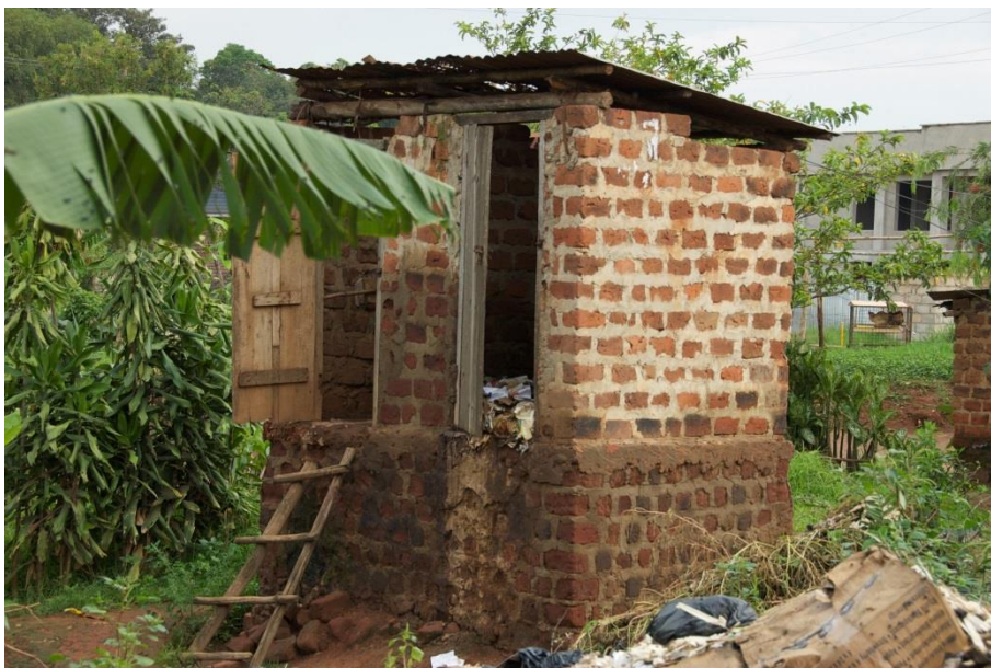
Figure 9: Damaged and abandoned pit latrine (Schoebitz, 2016).
