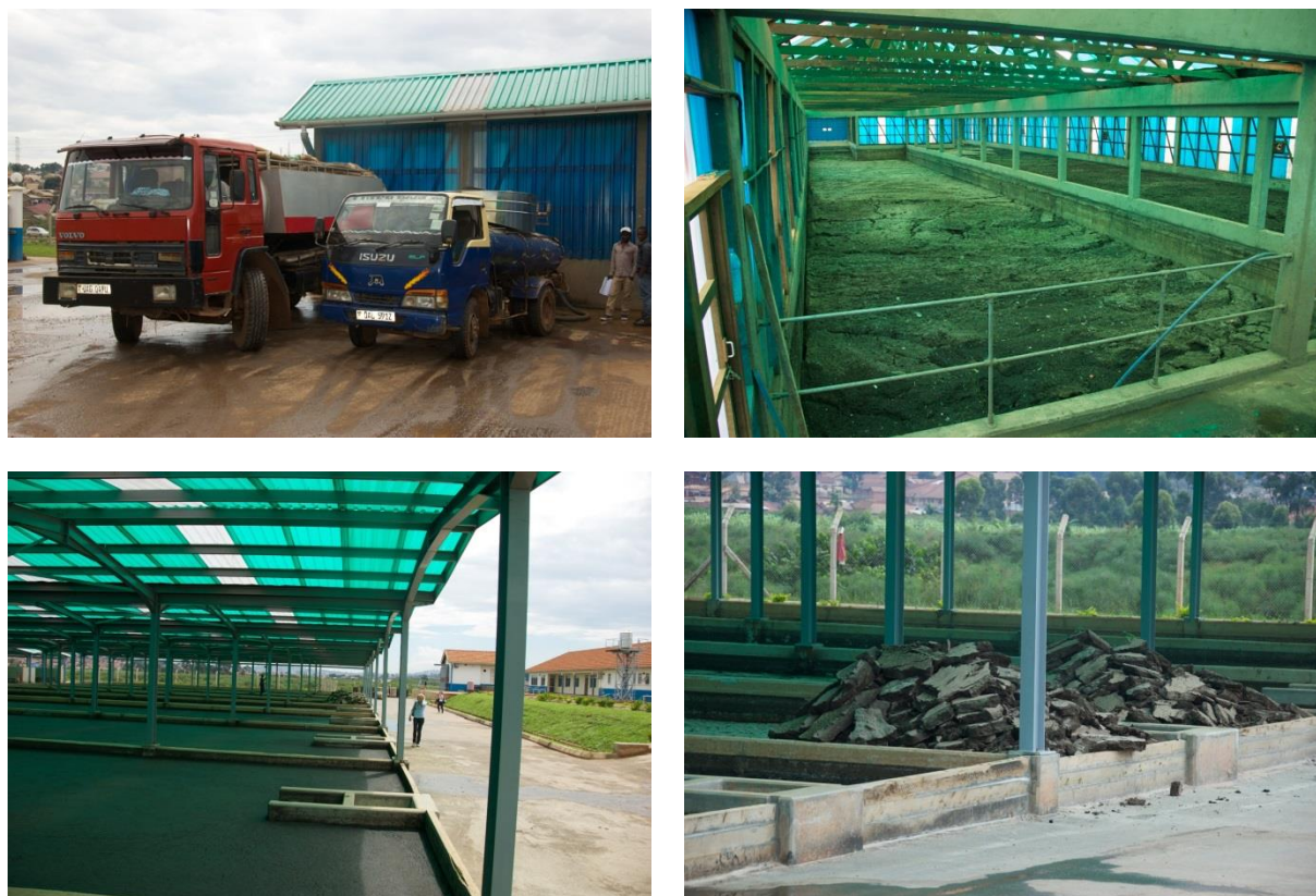
Figure 7: Lubigi wastewater and faecal sludge treatment plant. Top left: Discharge. Top right: Settling/thickening tanks. Bottom left: Drying beds. Bottom right: Dewatered faecal sludge. Photos (Schoebitz, 2016)
