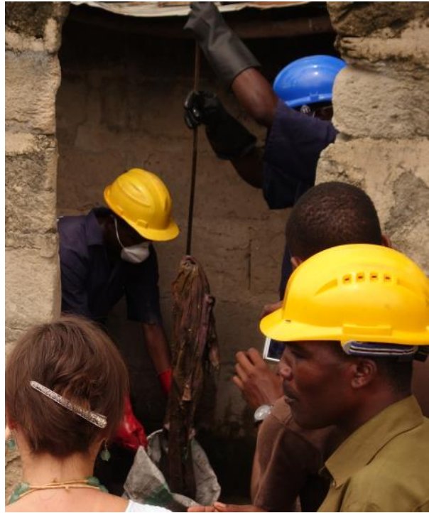
Solid waste removal from pit latrine before FS emptying. Photo credit: Imanol Zabaleta
