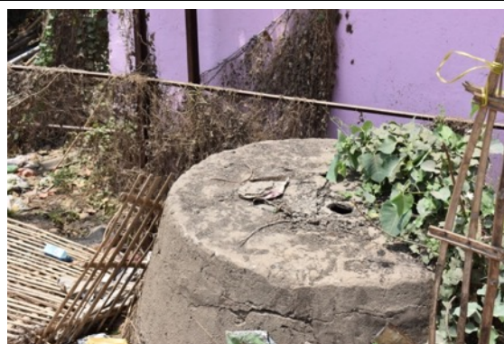
Decanting point outside the STP
