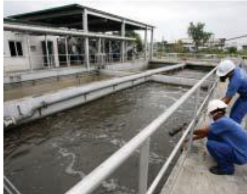
Figure 28. WWTP in Manila
