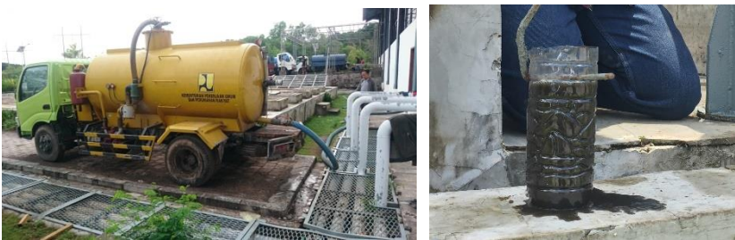
Figure 2. Poor effluent quality of treated septage due to ineffective septage treatment system – Effluent sample taken from a septage treatment plant in Denpasar- Indonesia with a capacity of 400m 3 /day (Source: Author)
