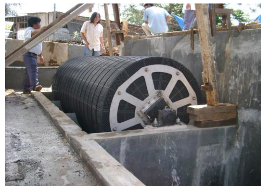
Figure 17. RBC with three-dimensional lattice contactors (Source: PUSTEKLIM)
