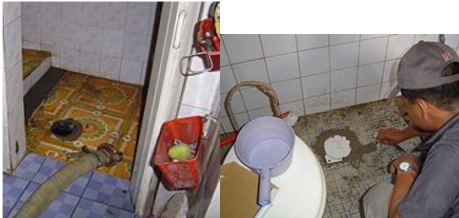
Figure 29. Worker installing a plastic cover to the access hole after septage emptying in Haiphong City (Source: 'URBAN DOMESTIC WASTEWATER MANAGEMENT IN VIETNAM', Water Environment Partnership in Asia)
