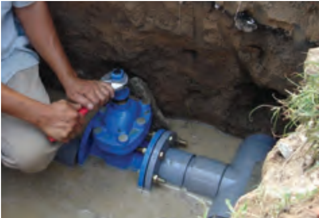
Broken pipe at a stop valve
