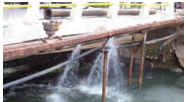
More obvious leaks
