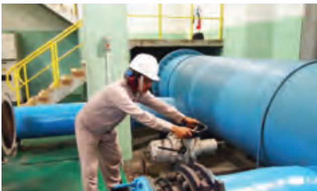
Valve turning under intermittent supply
