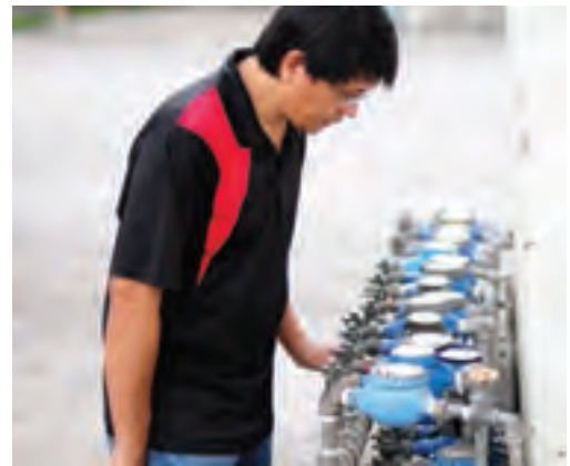
Customer water meters
