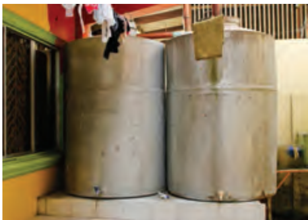
Rainwater harvesting tanks
