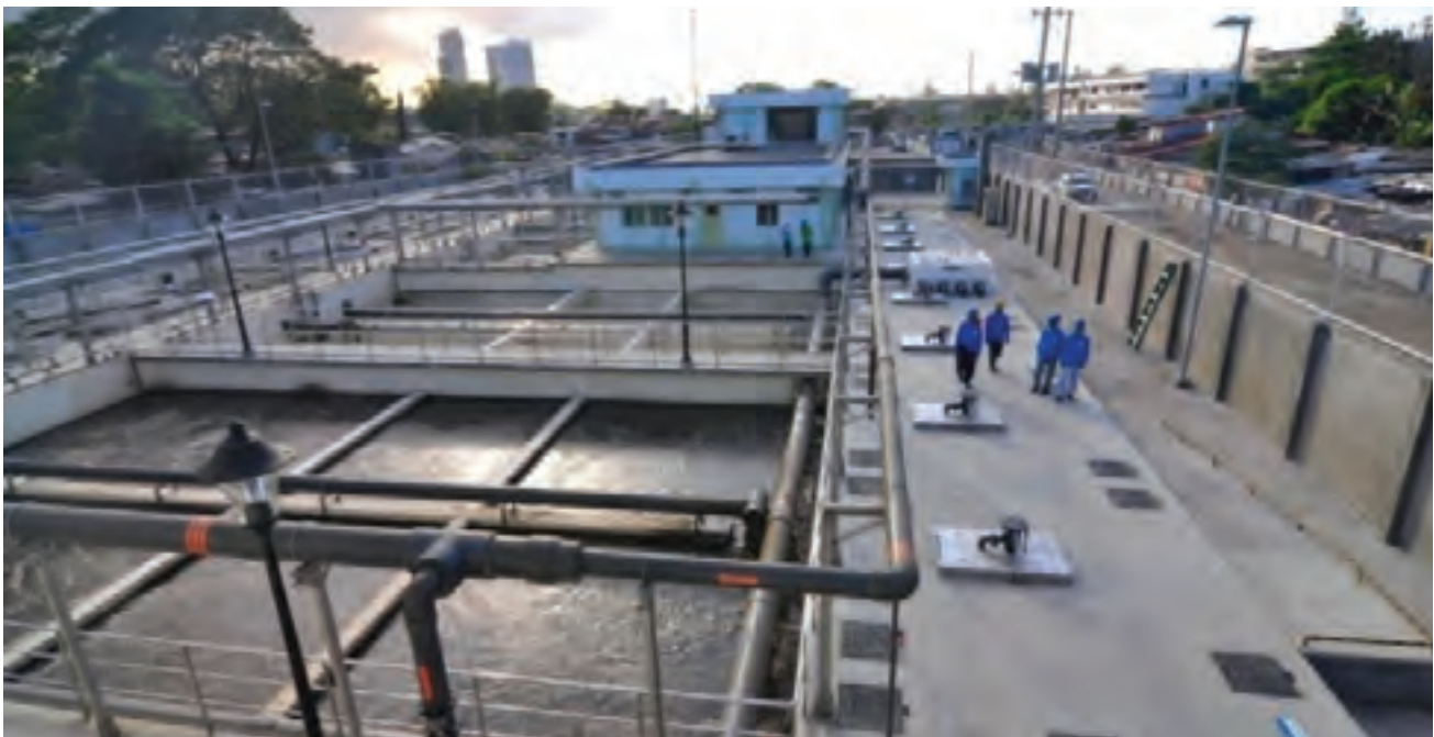
Sewage treatment plant in Singapore
