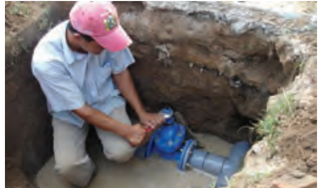
Closure valve on water network
