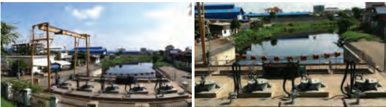
Sewage pumping station
