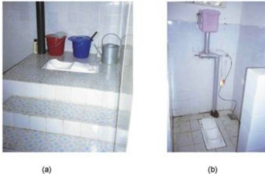
Figure 2.10. Urine-diversion ecosan toilets in Nanning area, China. (a) Toilet in a house. One bucket contains ash and the other bucket is for disposal of toilet paper, while the water can is used for rinsing the urine bowl. (b) School toilet. This version has a prototype ash dispenser. Ash or sand is stored in the "cistern" and depressing the foot-pedal spreads a small amount over the excreta deposited in the toilet. (Sanres 2000).
