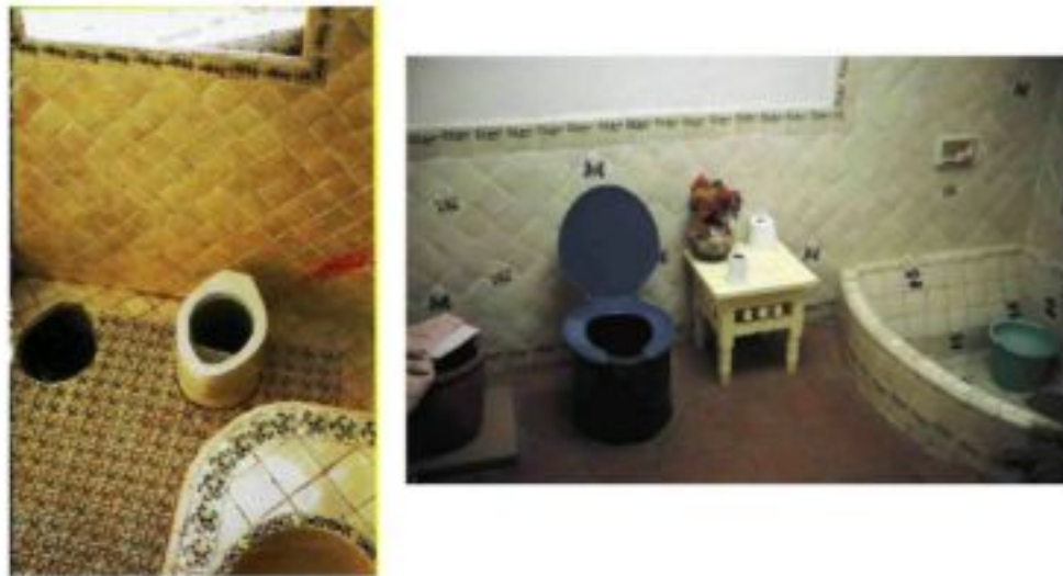
Figure 2.5: The Mexican version of the Vietnamese double-vault toilet, installed in the bathrooms of modern houses in the city of Cuernavaca. The toilets have movable urine-diversion pedestals. The processing chambers below the bathroom floor are accessible from outside the house (César Añorve, CITA, A.C., Mexico)
