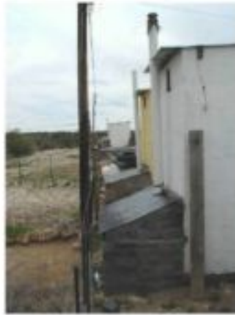
Figure 2.16: Conversion of bucket toilets in Campbell, Northern Cape (Photograph: R. Holden, Mvula Trust)
