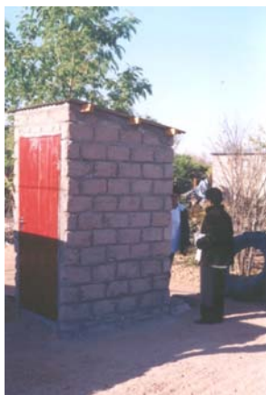
Picture 6: UD toilet in Augrabies (NC)
