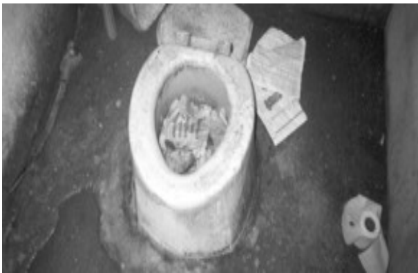
Overflowing VIP latrine
