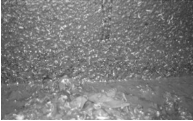
Walls of pit during emptying. This pit contained a very high load of maggots due to the fact that the ventpipe was missing.
