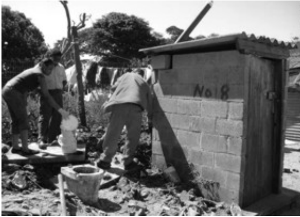
Project team standing by to take samples from different depths within the pit
