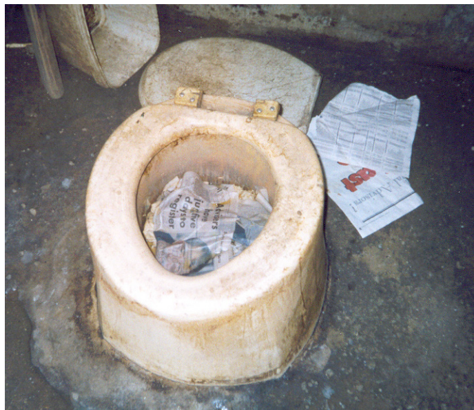
Figure 1.1: Photograph of a poorly maintained, overflowing pit latrine, filled with non-biodegradable material.
