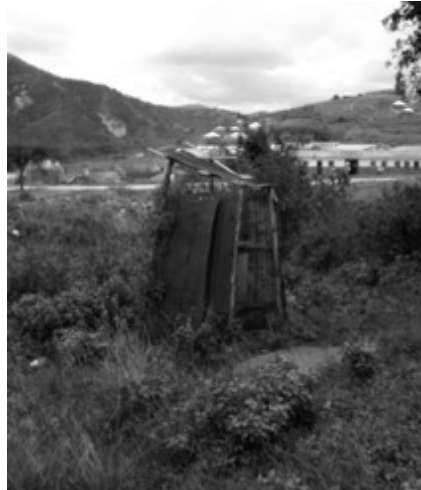
Rudimentary pit latrine with rickety superstructure in Maphephetheni
