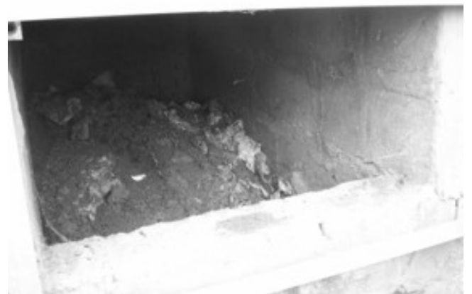
View into a half-filled vault of a double vault urine diverting VIP. The vault is mostly above ground.
