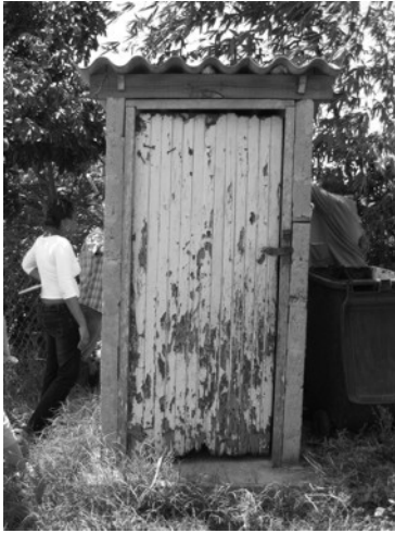
Poorly maintained community VIP in Tongaat area. This VIP had no vent pipe and the back plate was broken
