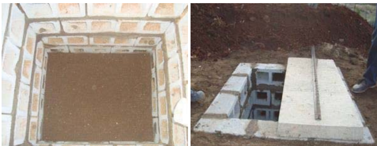
Figure 31: Soak pits used with pour flush and low flush systems. In this case the blocks have been turned on their sides to aid percolation of liquid from the pit. If the blocks are laid conventionally then the vertical joints must be left open (i.e. not mortared). The gap between the pit walls and the in-situ soil should be filled with river sand, which helps with percolation and will also act as a barrier against migration of most pathogens.
