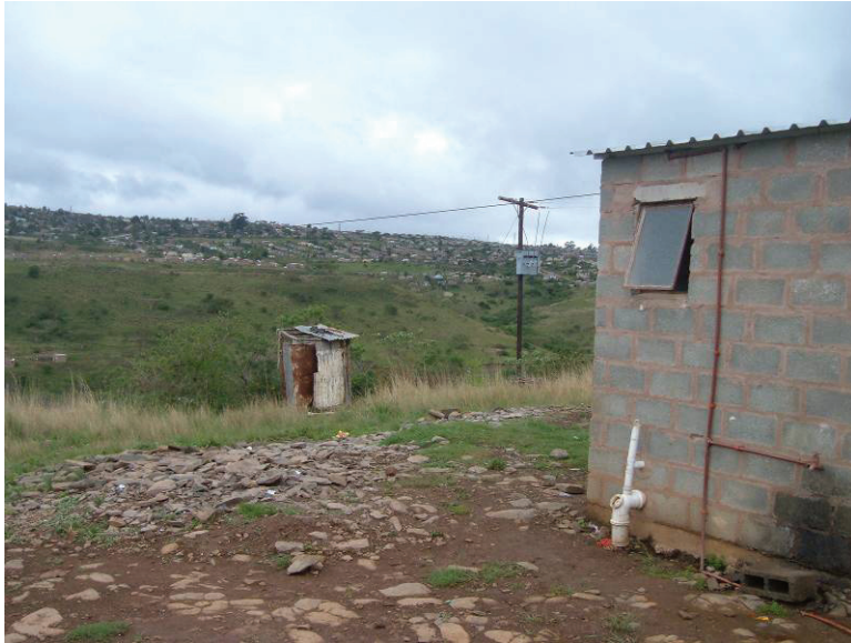
Figure 45: This family has constructed a VIP for themselves (background) as their flush toilet has failed due to the inadequacy of the septic tank and soakaway provided.
