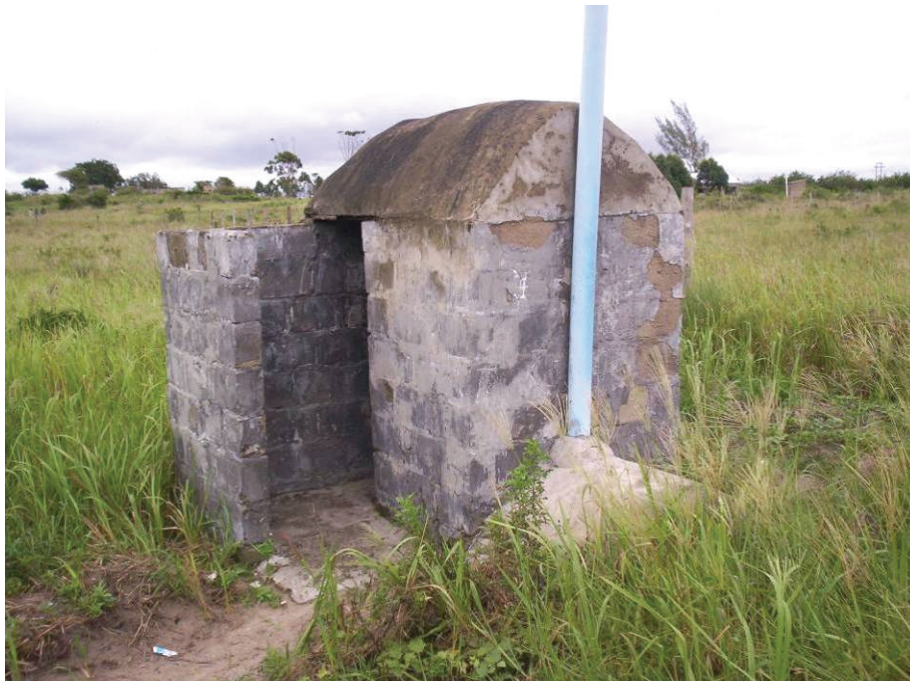
Figure 19: VIP toilet constructed in 1995 at Mbazwana northern KwaZulu-Natal (picture taken in January 2006)
