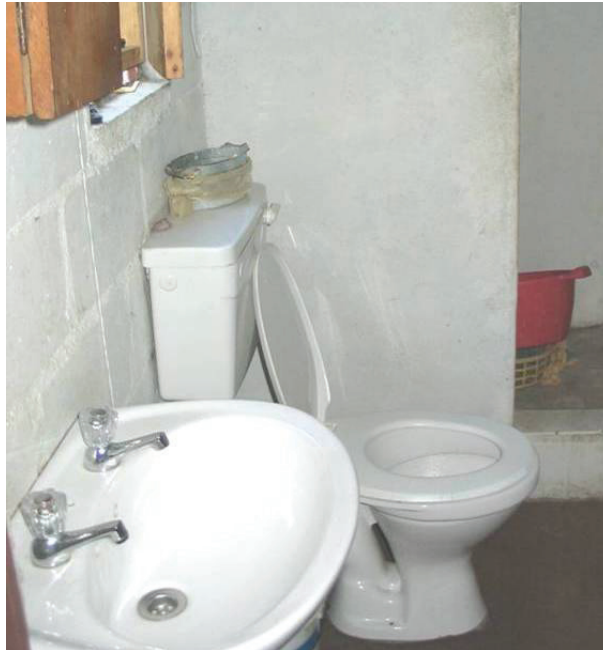
Figure 40: A well maintained indoor waterborne toilet on a Boland farm
