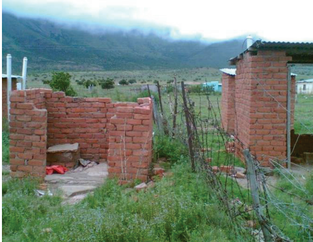
Figure 22: Damaged superstructure of VIP latrines in Thembaletu, Tsolwana Municipality, Eastern Cape
