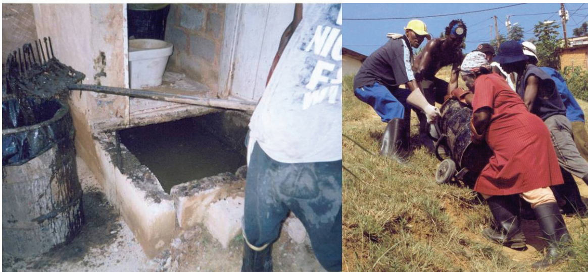
Figure 48: A labourer softening the sludge and removing the debris from the latrine, left; full tanks of sludge proved difficult to move up steep slopes, right (UWP, 2004)
