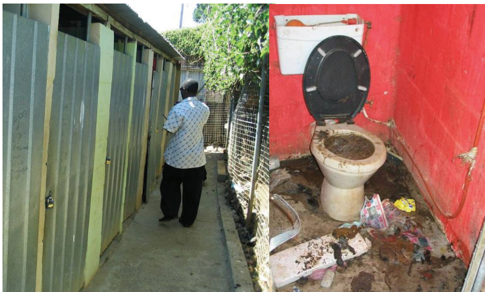
Figure 41: Block of waterborne toilets in Kayamandi (left), an example of communal waterborne sanitation where there is no defined person to clean (right)
