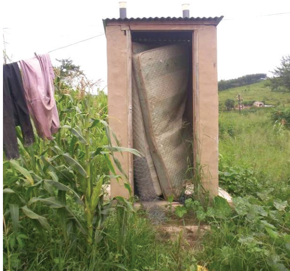
Figure 27: UD toilet with missing door being used for storage
