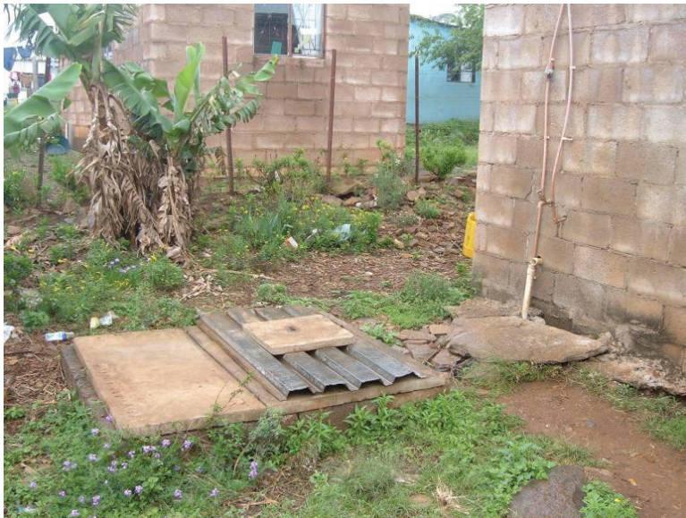
Figure 43: View of septic tank/soakpit combination used at Slangspruit in early phase
