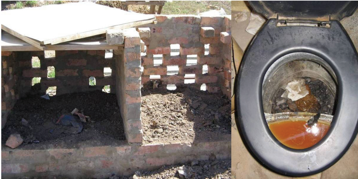
Figure 31: Composter at Bereaville, Western Cape (left); blocked urinal (right)
