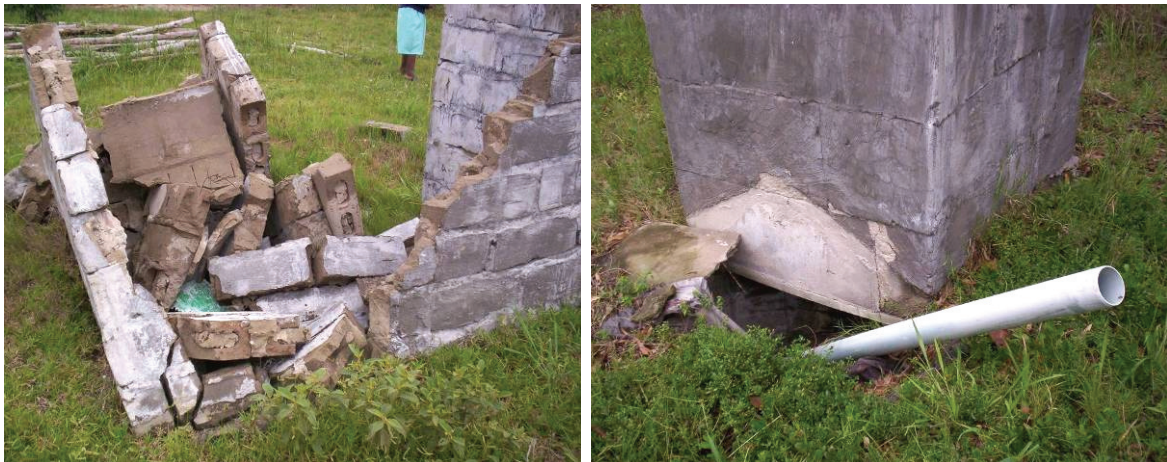
Figure 20: Collapsed VIP at Mbazwana northern KwaZulu-Natal (left); VIP toilet with a collapsed latrine chamber roof (right)
