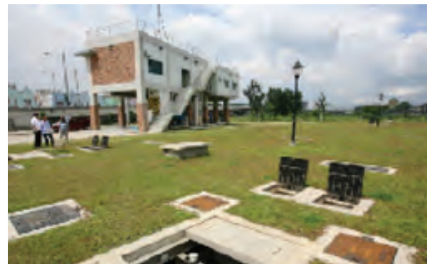
Olandes STP (Marikina City): process tanks built underground and support facility on stilts (Source: Steve Griffiths)
