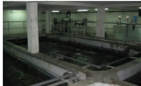
Pineda STP (Pasig City): aeration tanks under a basketball court (Source: Steve Griffiths)
