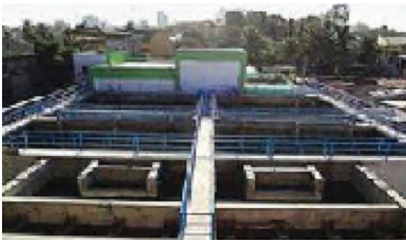
Moving Bed Biofilm Reactor (Paltok STP) (Source: MWSI)
