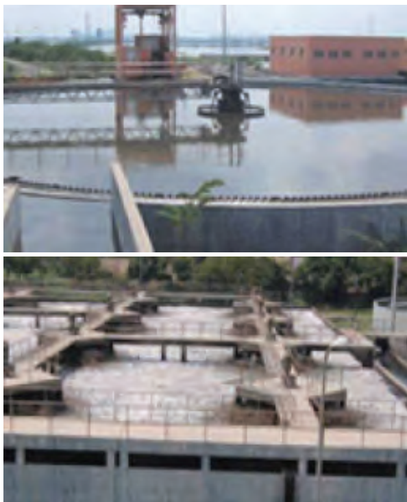
Wastewater treatment plant (Source: IWA)
