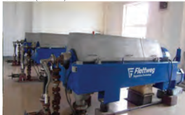
Sludge-Dewatering Centrifuges (Source: ADB)
