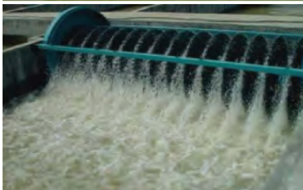
Xiang'an Sewage Treatment Plant (Source: Zhou Quilin)
