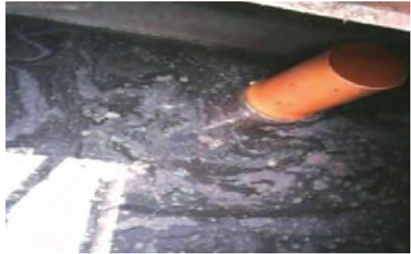
Wastewater in the anaerobic baffled reactor (Source: USAID-LINAW Project)
