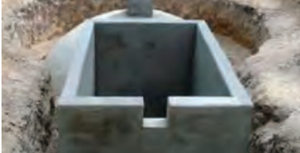
A nearly completed biogas digester, showing the mixing tank (rear), biogas digester (middle), and outlet (front). (Source: National Biogas Program, 2011)
