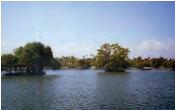
Wastewater treatment ponds: “Eco-Lagoon” (Photos: M. Ebarvia)
