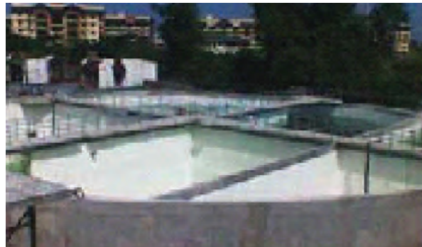
Sequencing Batch Reactor (Bagbag STP) (Source: MWSI)
