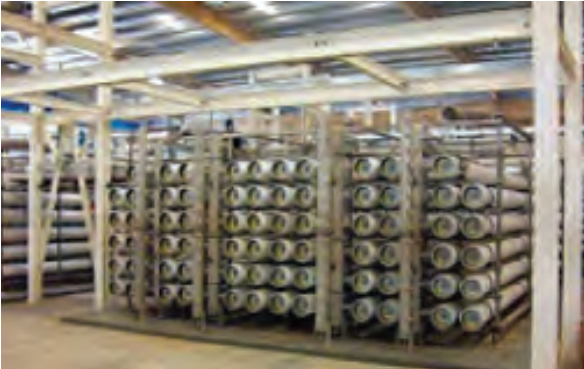
The plant has a total ultrafiltration (UF) membrane area of 304,640m 2 arranged in 68 skids. (Source: IWA)
