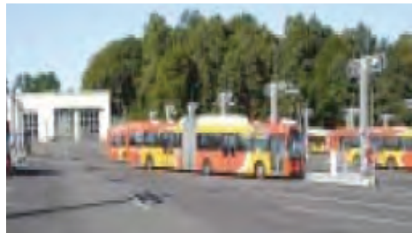
Slow filling system for city buses (Source: Svensk Biogas)
