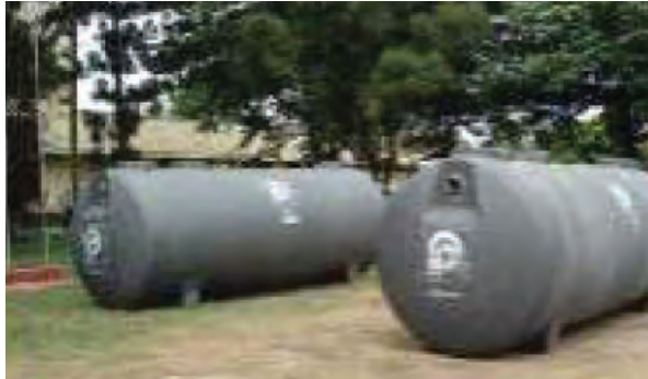
Eco Tanks (Source: Citynet)
