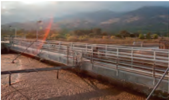
Fillmore MBR unit (Source: Mark Strauss, American Water Enterprises)
