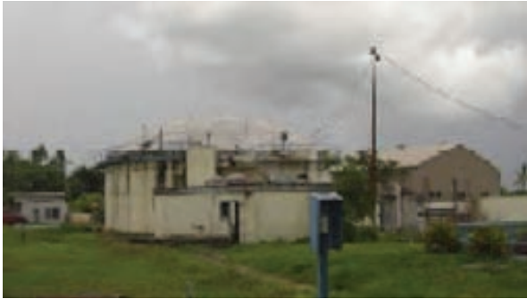
anaerobic sludge digester (Source: ADB)
