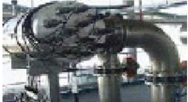
Ultraviolet disinfection (Source: PUB Singapore)
