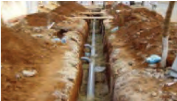
Sewerage system (Source: Viet Anh Nguyen)
