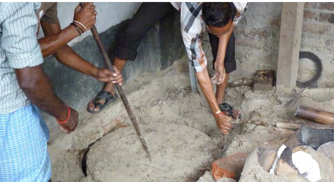
Figure 1. Municipal workers assist a homeowner in finding and uncovering the tank access for desludging.
